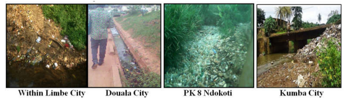
Figures 7 Urban drainage systems choked by waste to highly reduced water carriage potentials
